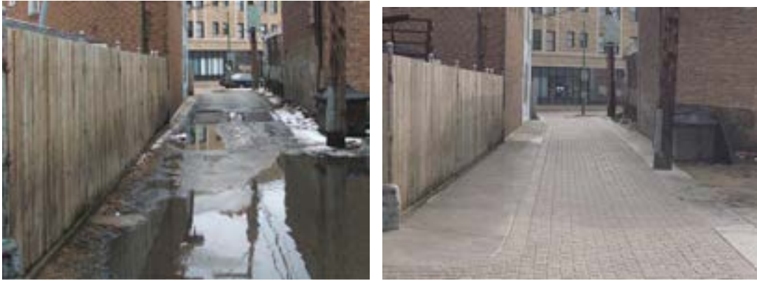
FIGURE 18. ALLEY WITH IMPERMEABLE PAVEMENT AND POOR DRAINAGE (LEFT) AND ALLEY INCORPORATING GREEN ALLEY PRINCIPLES (RIGHT) (CDOT).
